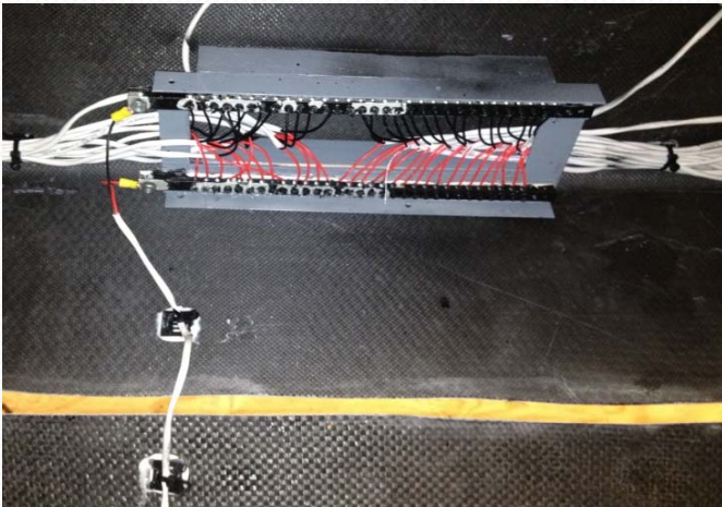
Solar Wiring Bus
